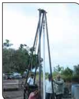
Lower Idol Column Pipes with Chain Pulley
