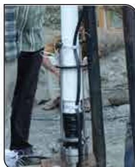
Ensure Pump Guard is Installed Properly
